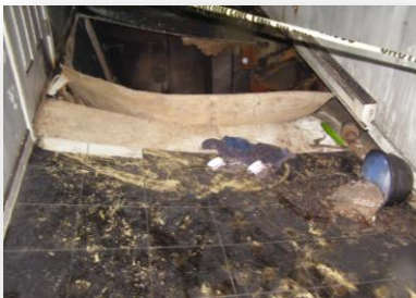
Image of the hole into which a firefighter fell, claiming his life, following the failure of engineered wood I-joists. (NIOSH Report 2006-24)
