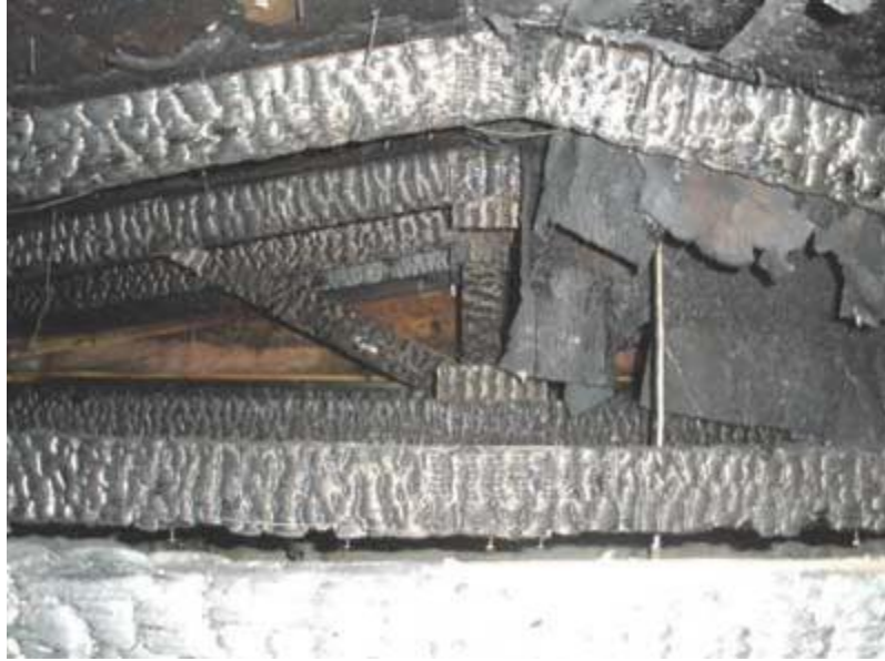
Modern lightweight metal gusset truss roof—with ceiling. Collapse Time = 23:15. (9) Multiple metal gusset plate and web member failures.
