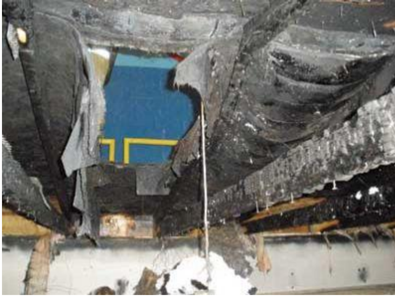
(10) The deterioration of roof sheathing and ultimate failure of the roof sheathing and shingle materials.
