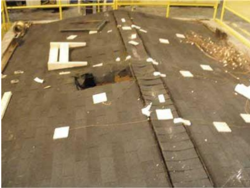
(8) The collapse of the continuous plastic ridge vent.
