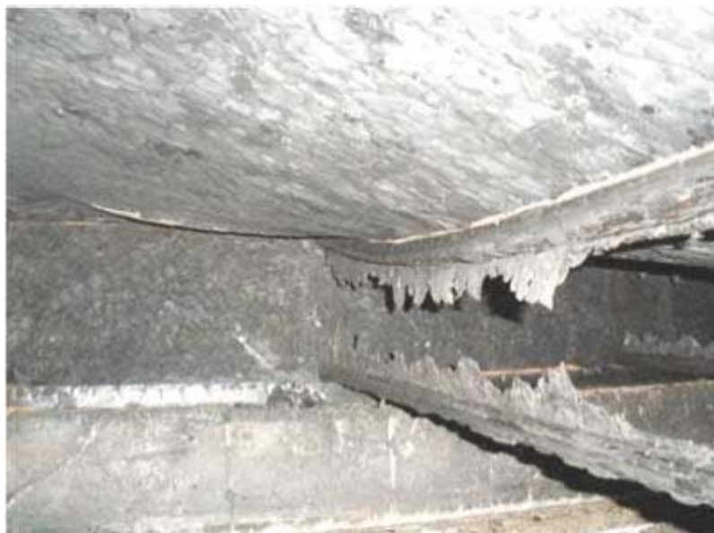
(6) Modern lightweight metal gusset truss roof—with ceiling. Collapse Time = 23:15.
