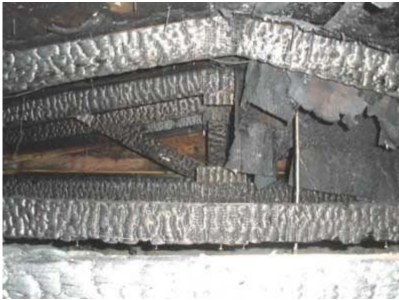
Modern lightweight metal gusset truss roof—with ceiling. Collapse Time = 23:15. (9) Multiple metal gusset plate and web member failures.
